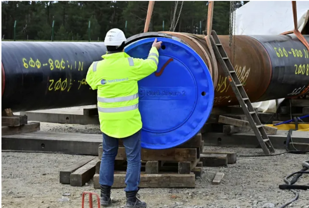
The Nord Stream 2 gas pipeline in Lubmin, north-eastern Germany © AFP via Getty Images
