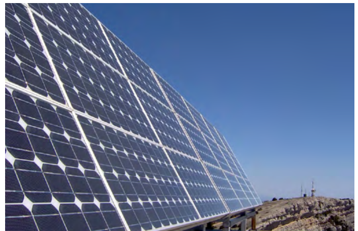
Some small-scale distributed solar plants will gain access to SGCC’s power grid. (Flickr)
